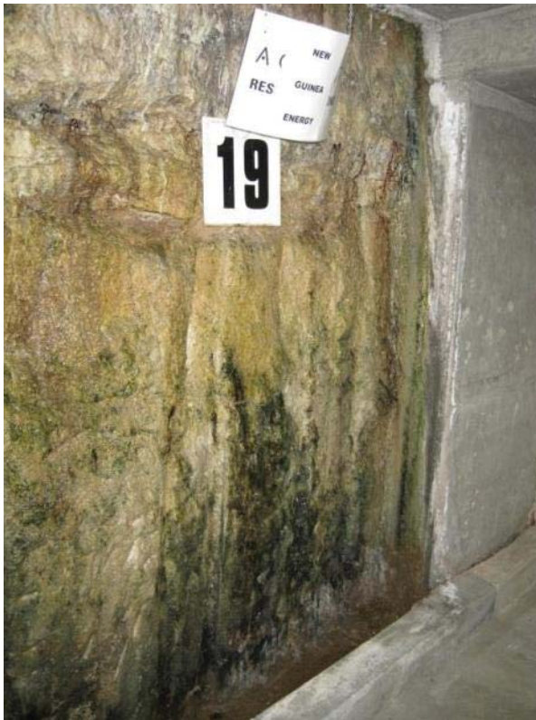
Figure 9 Groundwater seepage 2-10 Loftus Street
